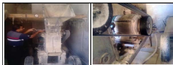
Fig. 2. The mill grinding machine Fig.3.The electrical motor.
